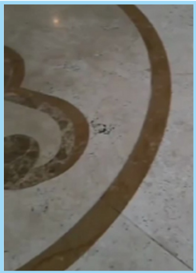
Before repair: damaged weathered stripper cracking
